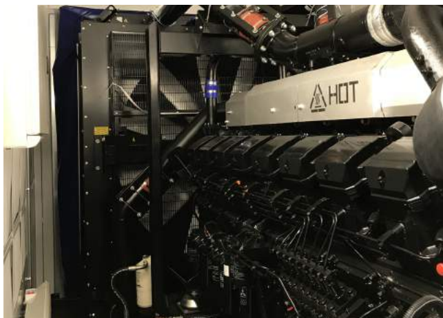
The T2200 Kohler-SDMO generator set positioned within the bespoke acoustic enclosure.
