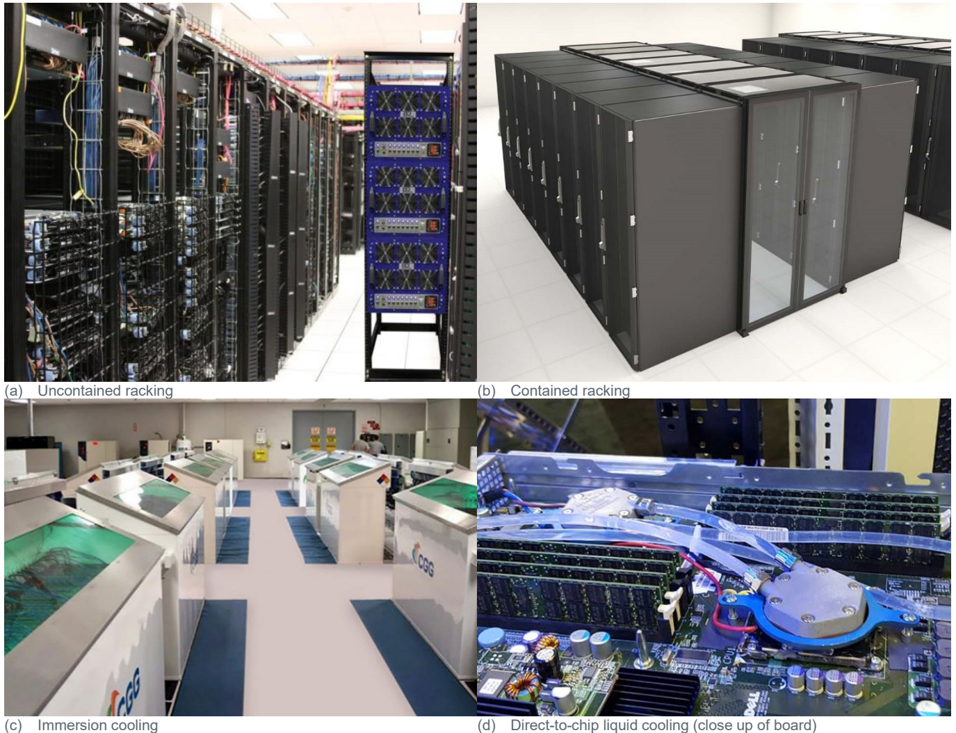
Figure 3: Examples of air- and liquid-cooled server racks
