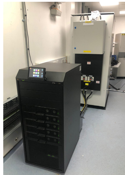
UPS & battery cabinet
